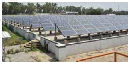
Solar Panels at Sahiwal Factory
